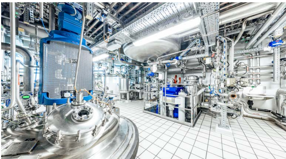
The latest reactor systems reflect the company's technological leadership.
